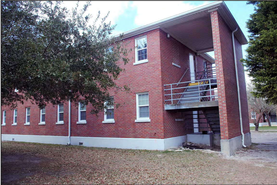
PLATE 18: RR5, South Elevation, Showing Exterior Stair System Renovation from 1970s-1980s, Stone Bay Rifle Range Historic District, Camp Lejeune, North Carolina
